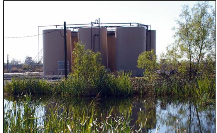
East Chalkley Tank Battery
